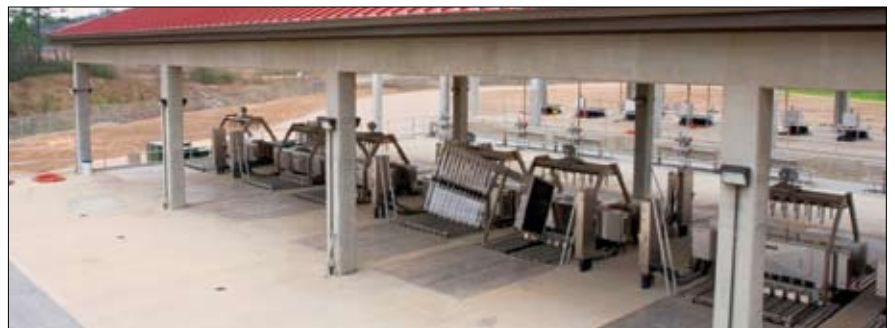
The eight TrojanUV4000Plus™ reactors used to disinfect 600 MGD (94,680 m 3 /hr) at this large wastewater treatment facility require a footprint measuring only 80' x 120' (24 x 36 m) – a fraction of the space needed for chlorine disinfection.
