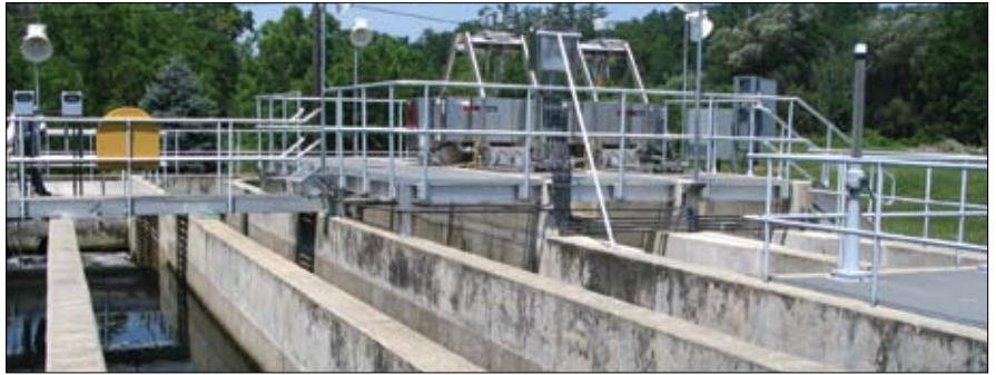
In this retrofit installation, each reactor was installed in one pass of the existing chlorine contact basin with only minor modifications to the channels. This allows the majority of the basin to be used for storage, by-pass or emergency back-up.
